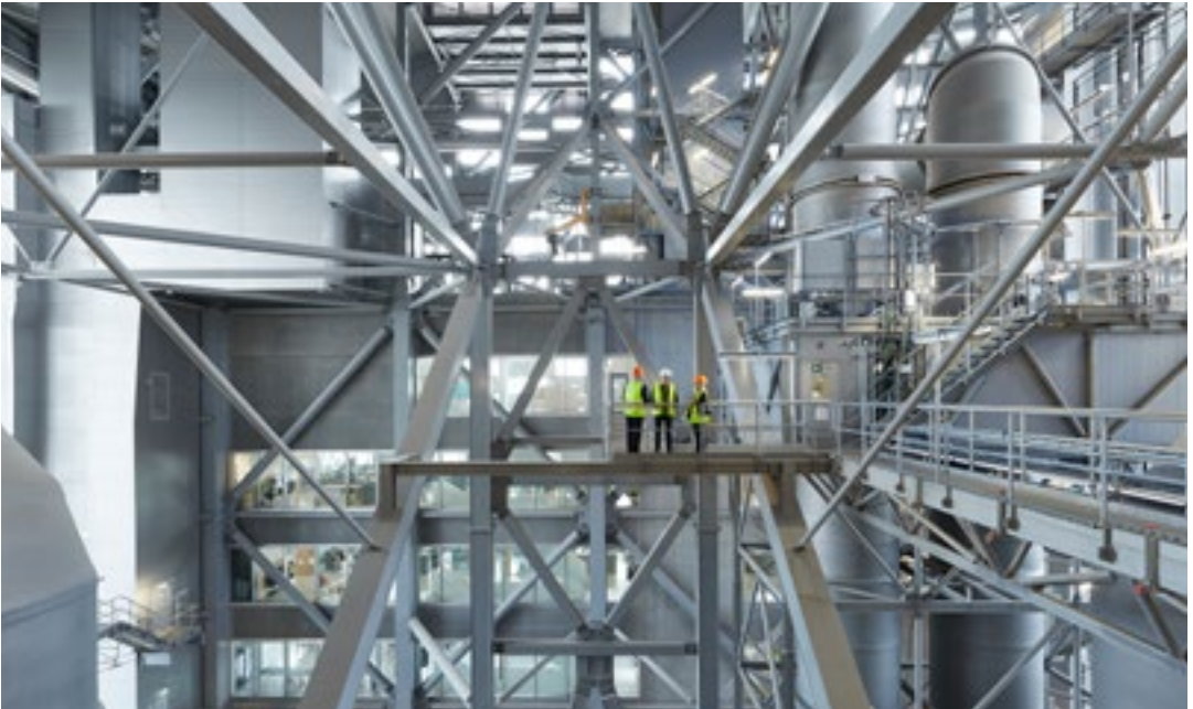
Inside Copenhill, modern waste treatment machinery is all arranged in height order, which forms the building’s sloped rooftop and resulting 9,000-metre-squared ski and recreational terrain. Photograph by Soren Aagaard
